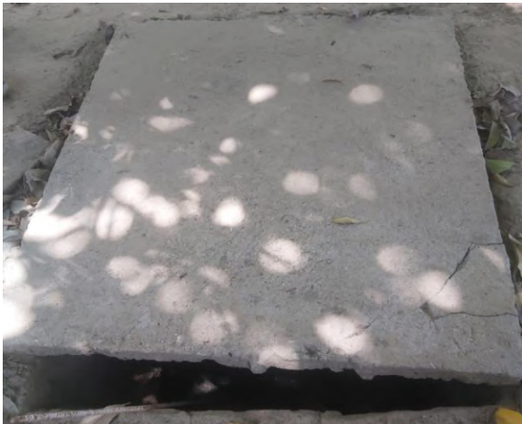
Wastewater collection tank
