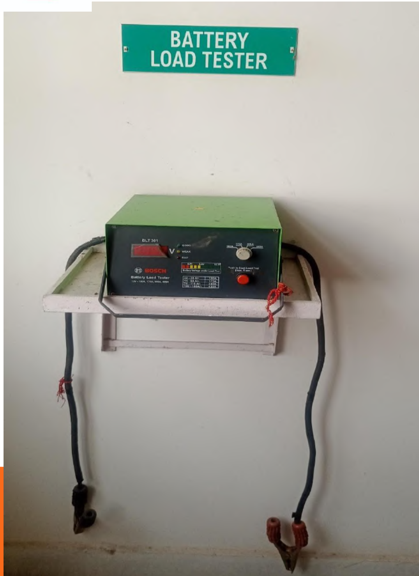
BATTERY LOAD TESTER
